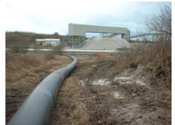
Part of the 560mm PE100 SDR17 pipeline which runs beneath the River Weaver.
